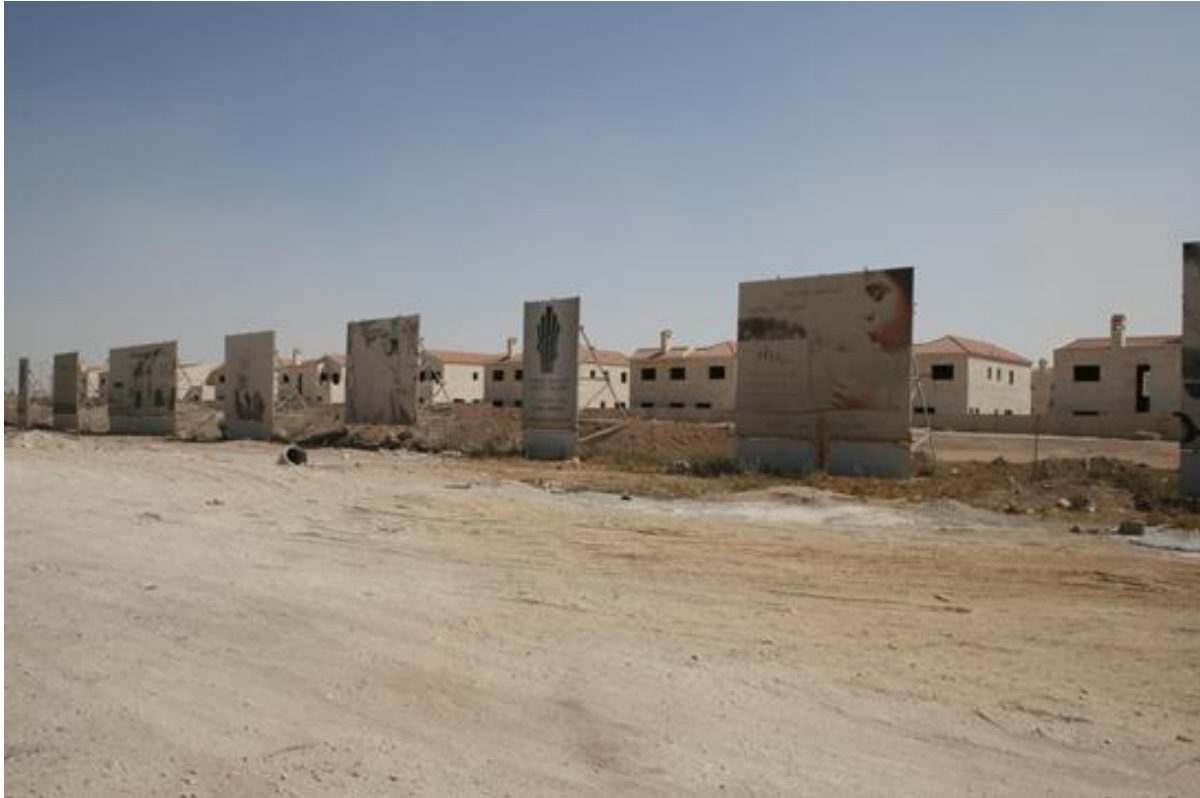
Fig. 2 - The gated community site of Andalusia on the Airport Highway. (Photo Credit: Rami Daher)
